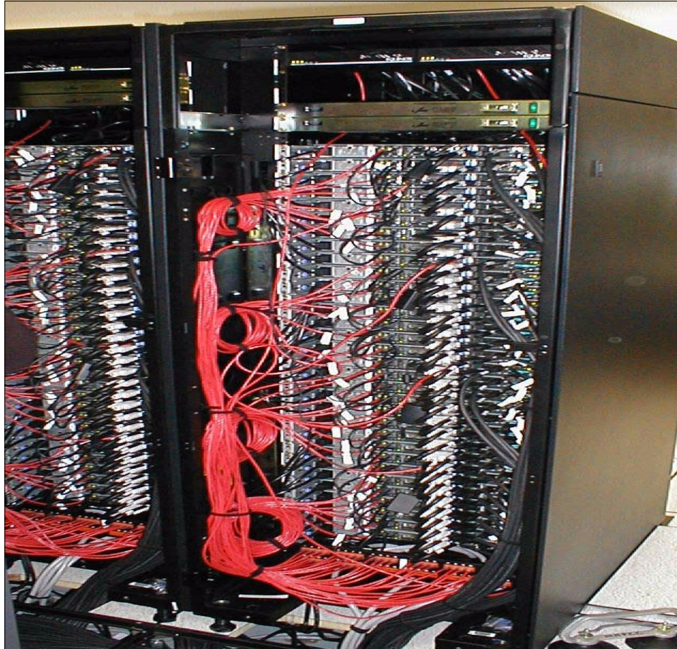
Figure E-3 Ethernet cables
