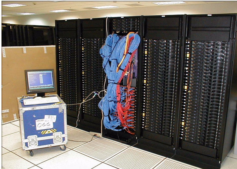
Figure E-2 Fibre cables
